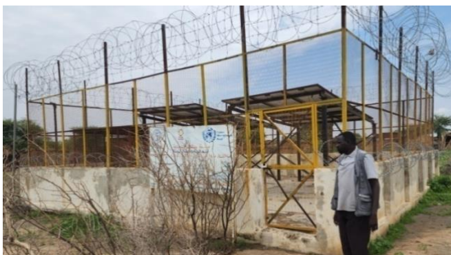
Plate 5h: Hybrid system at Kass to operate water supply system
